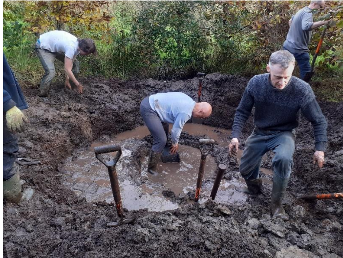
Figure 4 Pond construction at October Wood: never happier than when we are working in a muddy hole.
