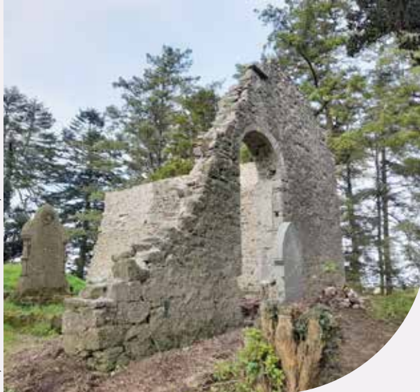
Derryvullan Old church Ruins funded by the Landfill Communities Fund
