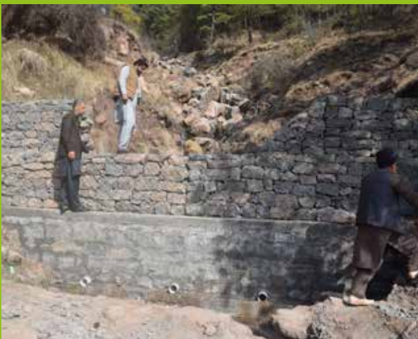
One of the dams we built in Azad Jammu and Kashmir to better protect homes and livelihoods.
