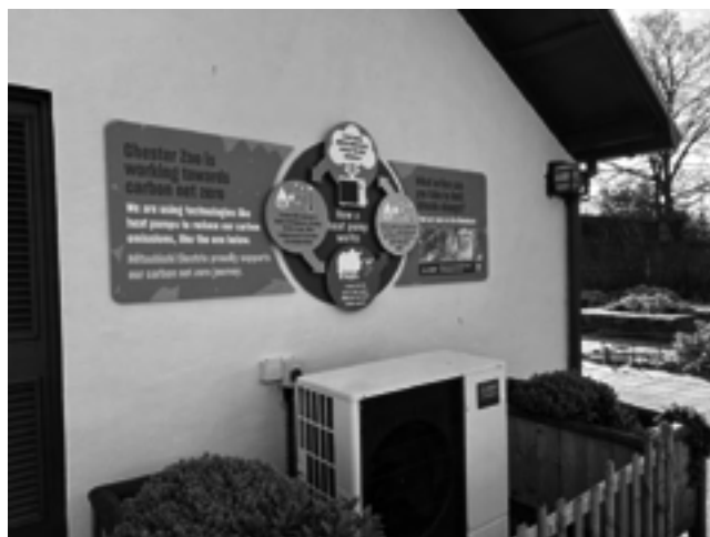
Educational signage about our partnership with Mitsubishi Electric and our use of air source heat pump technology on-site to decarbonise our heating.
