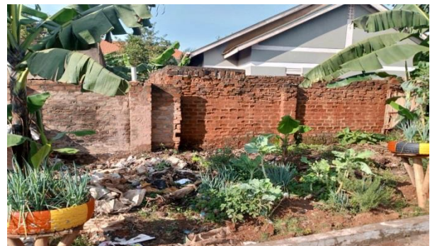
Rainfall slowly eroding away the unplastered bricks
