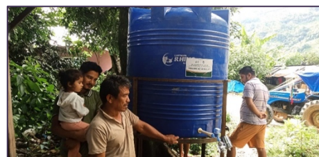
Water harvesting, storage, and filtration installations
