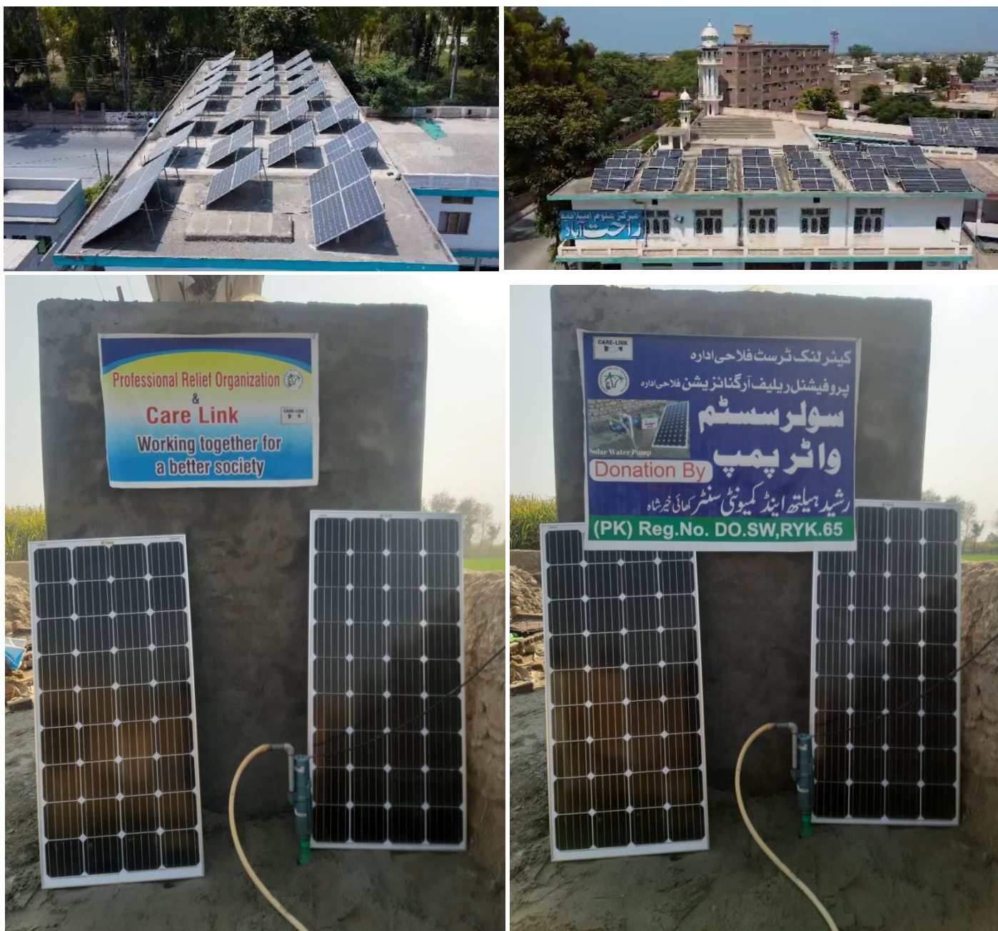
Figure 11: Solar Panel System- Ziyara, Layyah, Akorha Khatak
