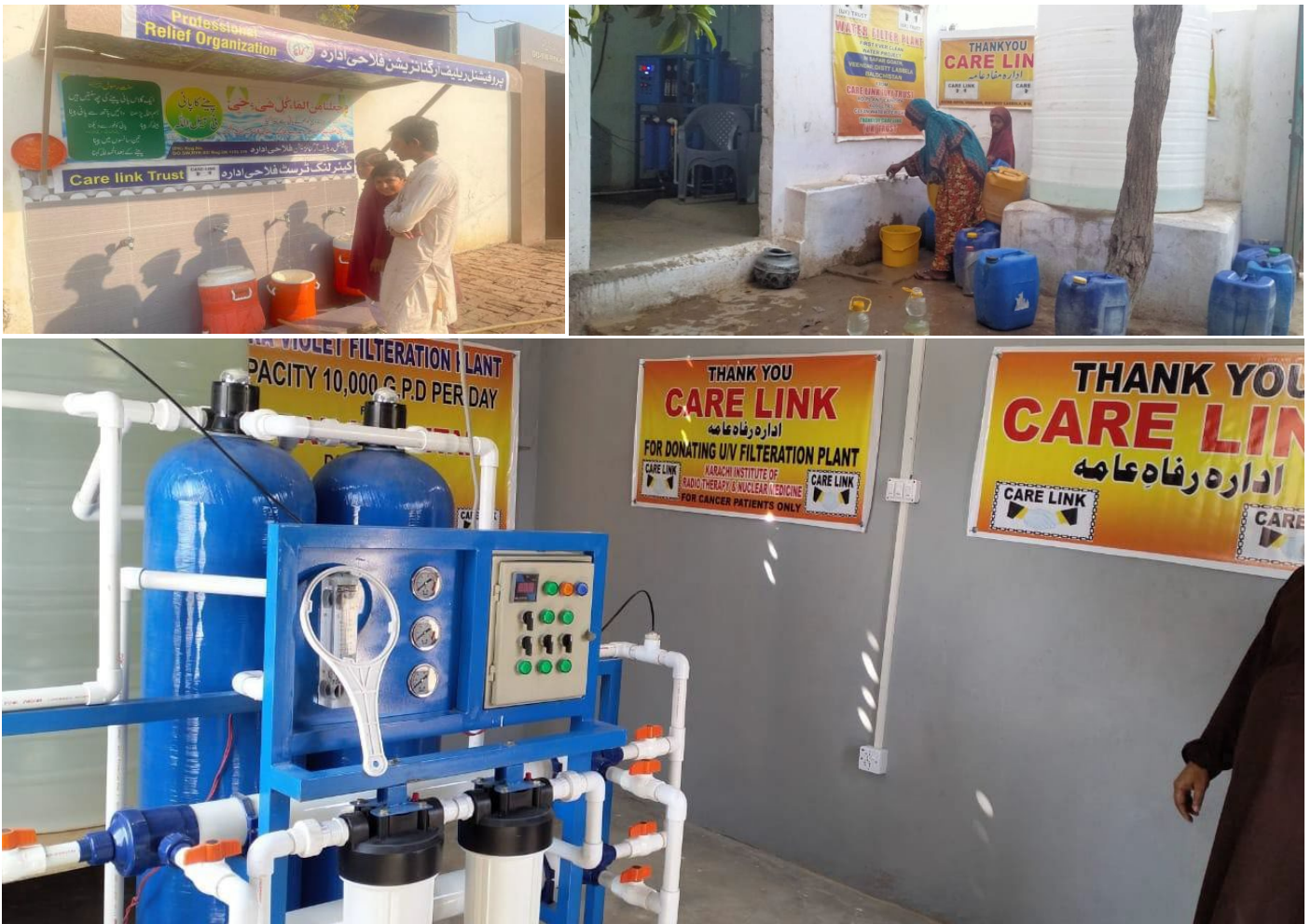
Figure 6: Water Filtration Plant – Vinder Balochistan
