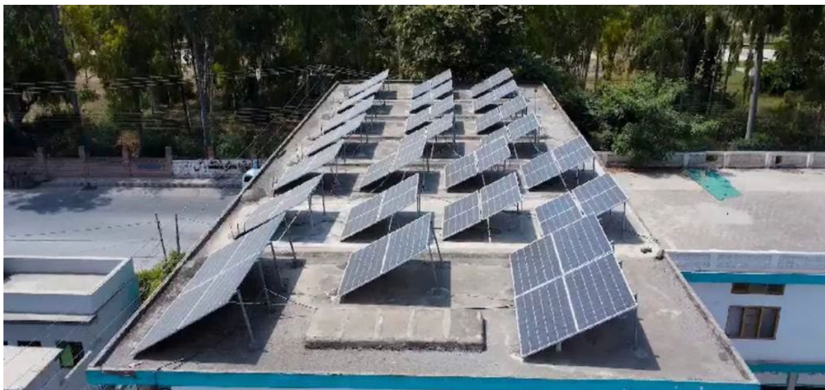
Figure 12:CLT Solar Project
