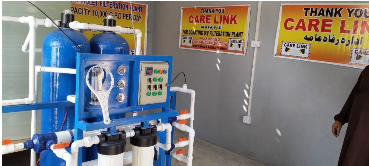
Water Filtration Plant in Karachi
