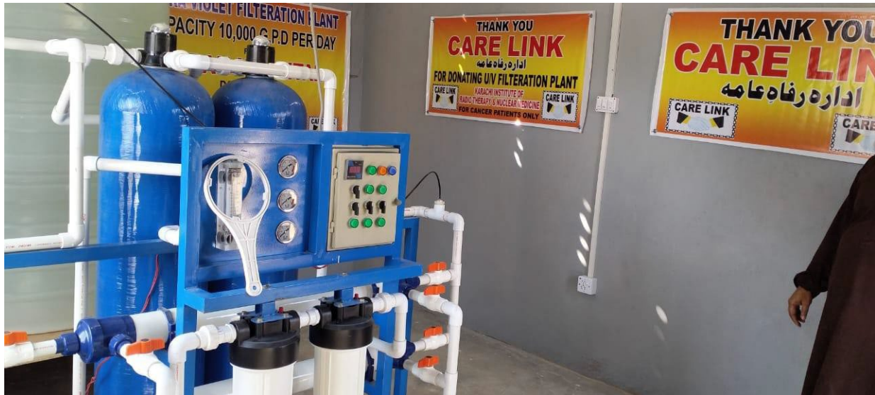
Figure 5: Water Filtration Plant
