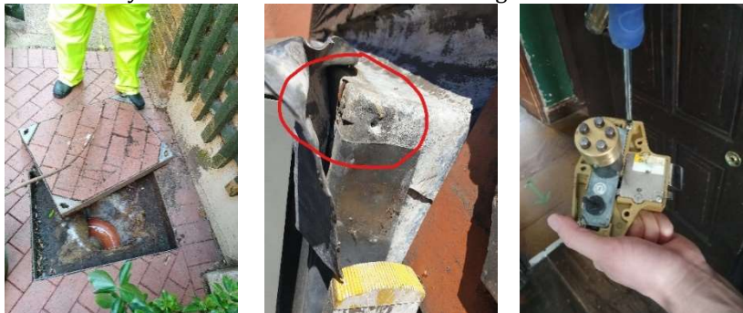
Example of in house repairs to faulty locks, cracked lead work and blocked drainage.
