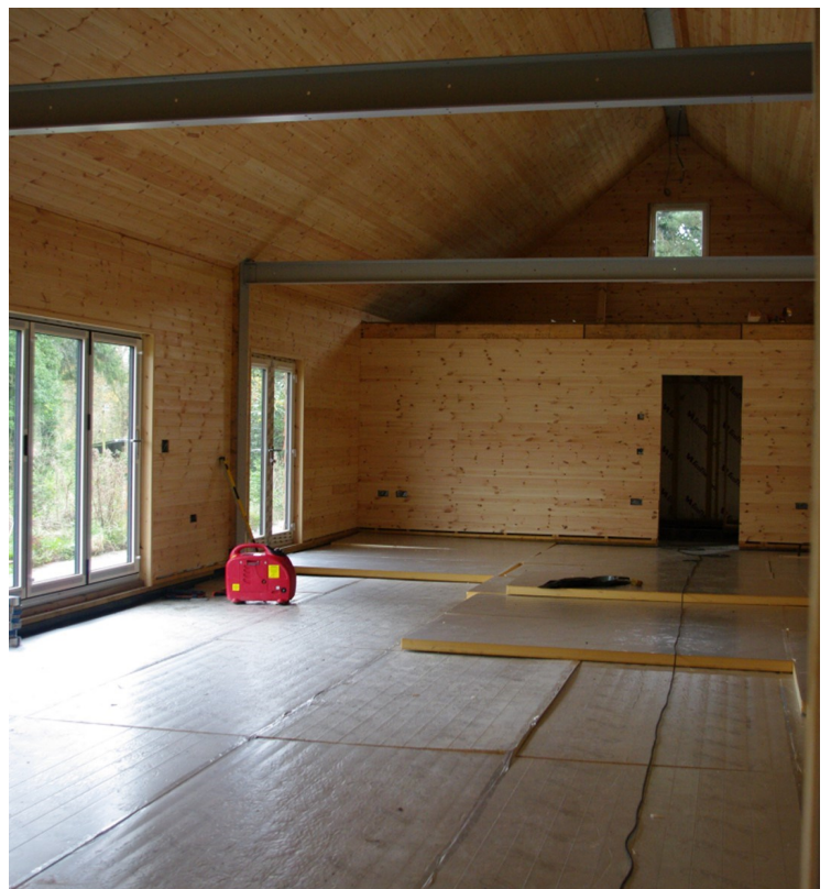
Inside cladding complete. Floor insulation going down. Next is the pipework for the underfloor heating.
