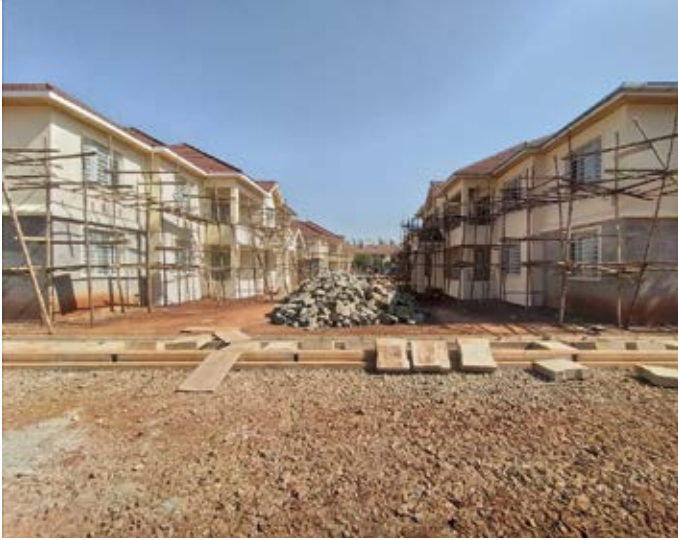
Construction of new officer accommodation (above) in Nairobi, Kenya, with groundbreaking plaque recognising IHQ funding support (right)
